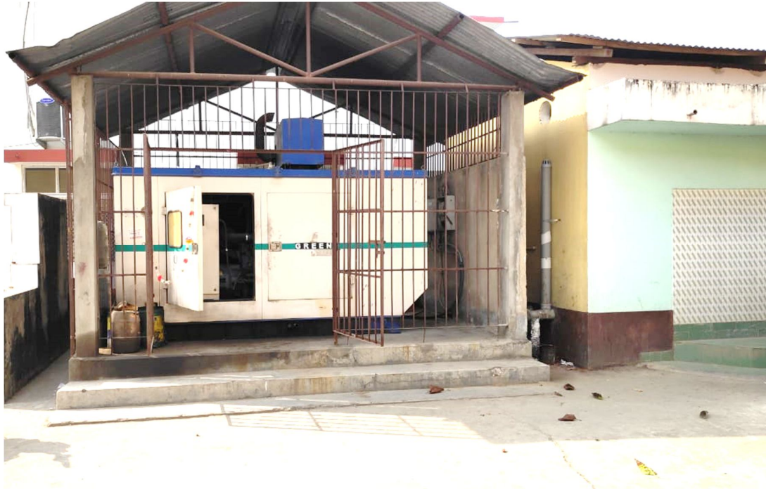
Figure 9 Diesel Generator Set
